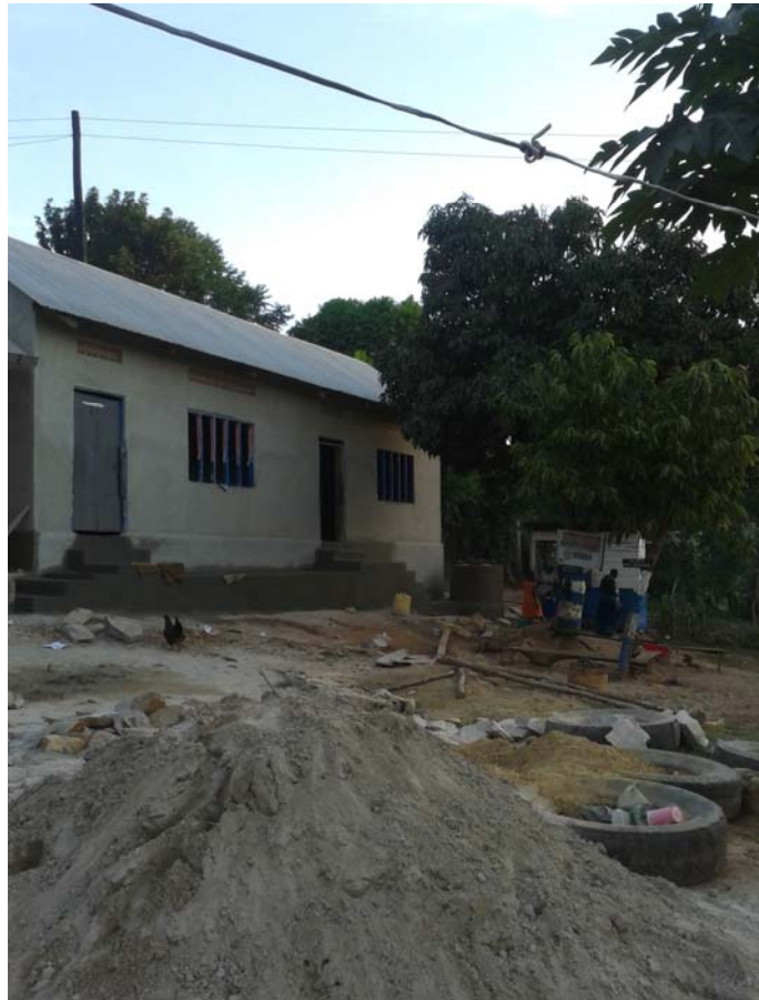
The exterior renovations are being completed on classrooms originally constructed by Project Kesho in 2008. (July 2013)
