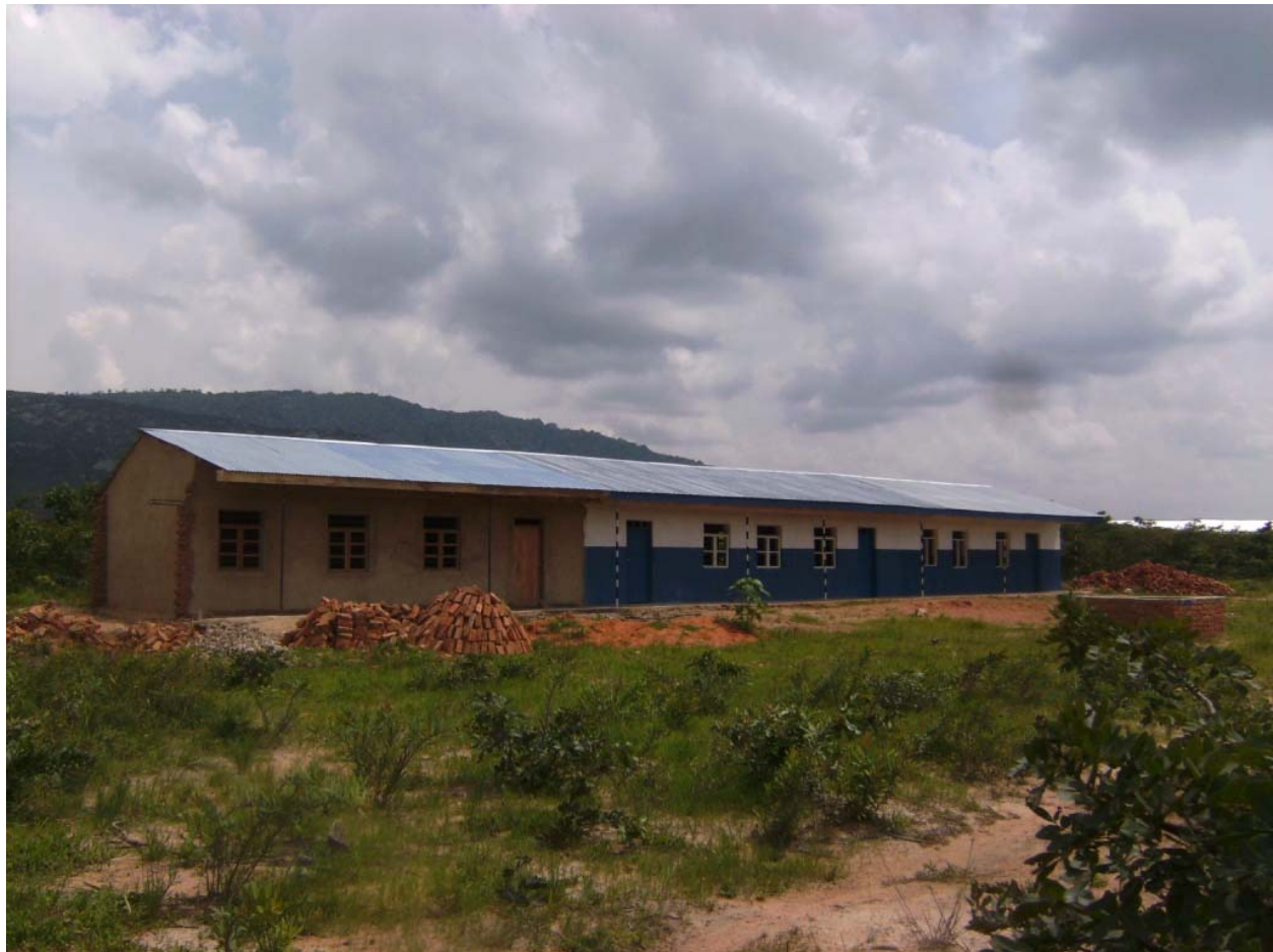
The third classroom at the new Kibati Primary School, just before receiving a coat of paint.
