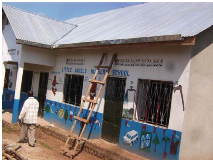
The new classroom building at Little Angels being fitted with gutters for rainwater harvesting.
