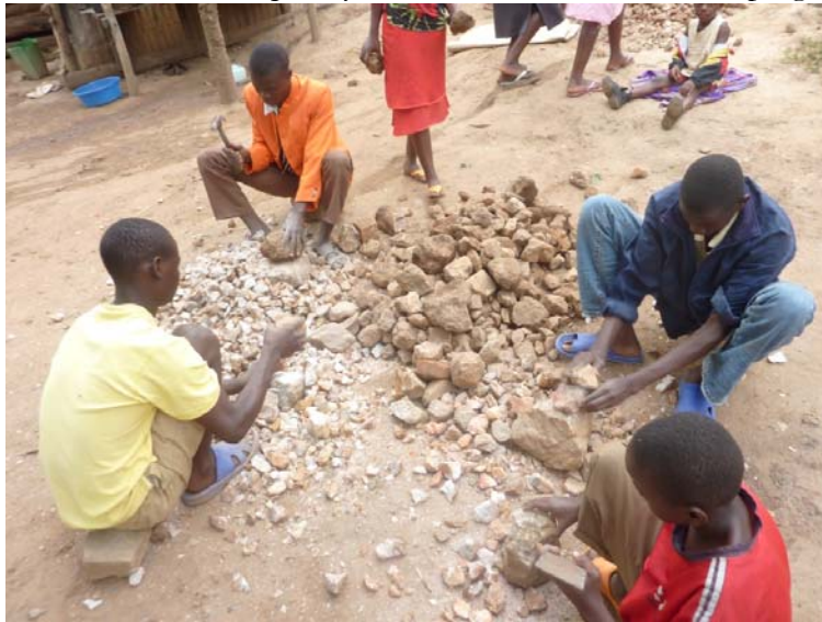
Breaking rocks by hand to be used in the foundation of new classrooms at Little Angels Primary School.
