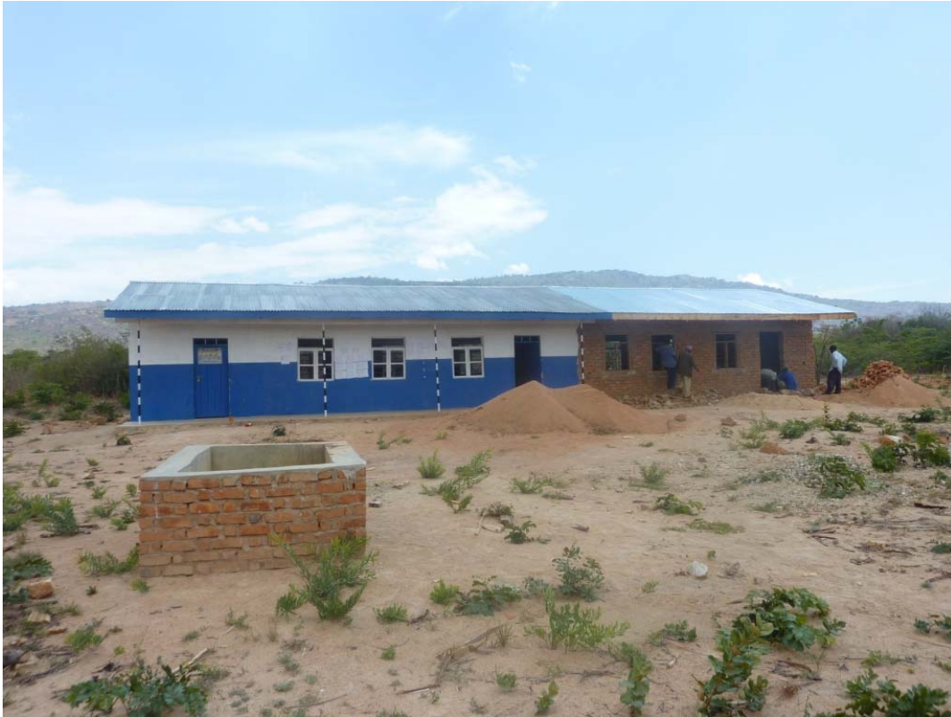
Work being completed on the second classroom at the new Kibati Primary School.
